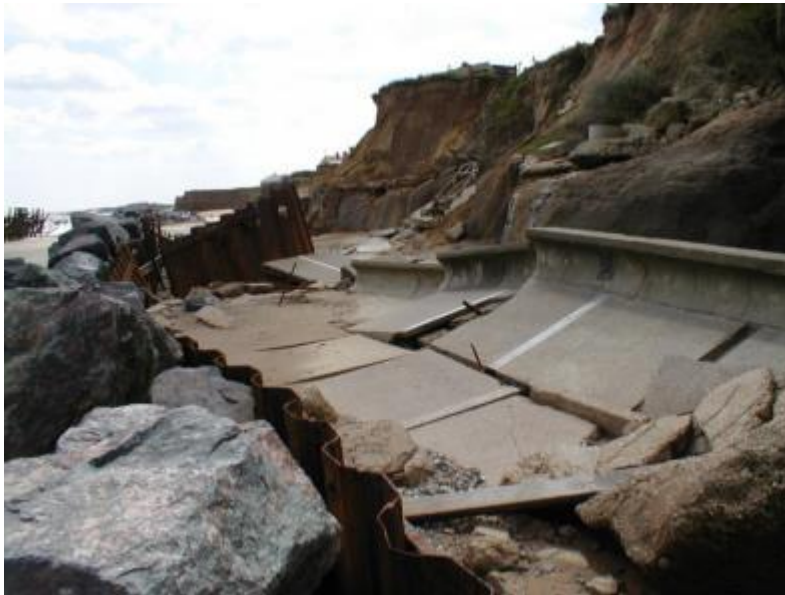
Failed sea wall at Happisburgh, Norfolk, UK
